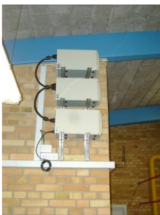
UPS-batterier for video-overvågning.
